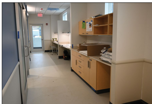
The walls have been painted and shelving is going up in our pharmacy hallway, which is part of the clinic space added to the front of our building.
